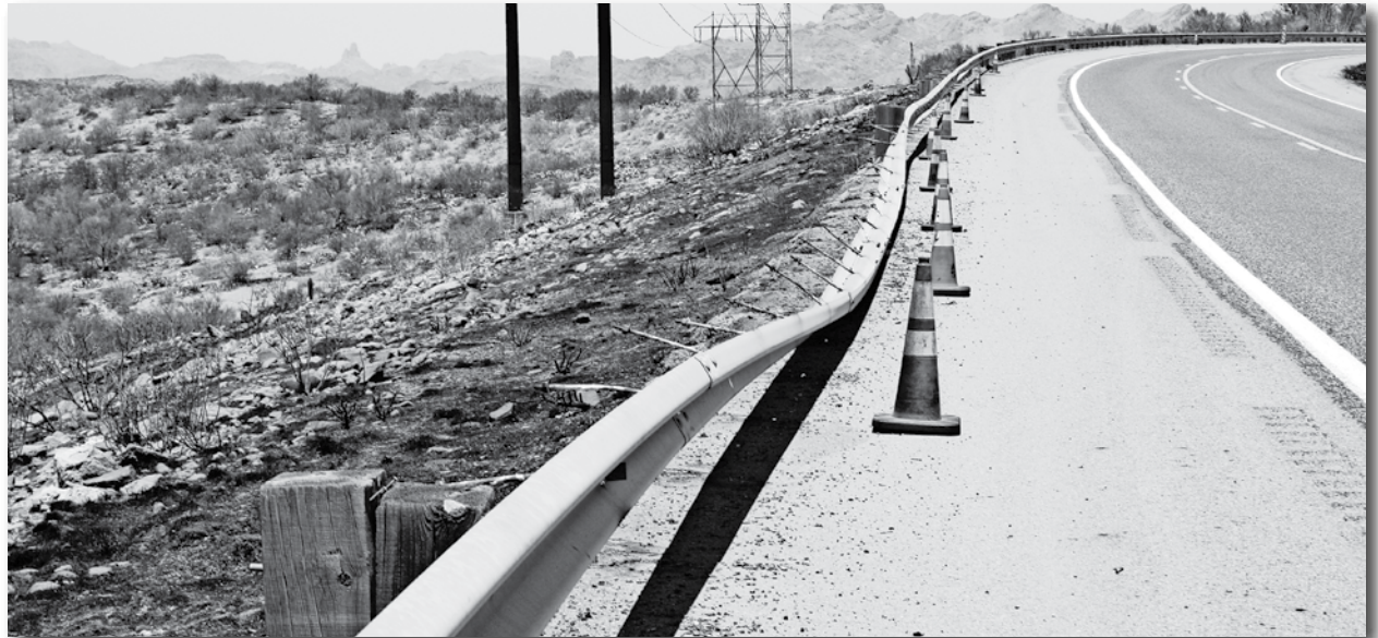
Drivers should be extra careful when Arizona Department of Transportation workers are replacing burned and damaged guardrails. James Carnes | CBN
