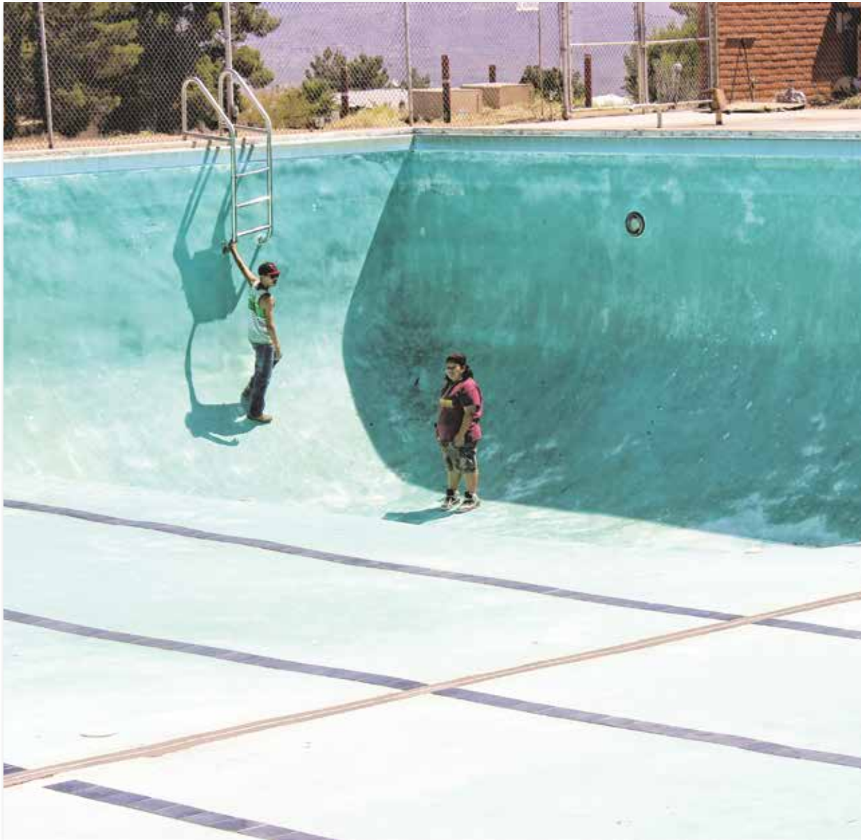
Volunteers Maurice Ochoa, left, and Lexus Buzan are amazed at the size of the San Manuel Pool. It looks so much bigger when empty. Other volunteers who are not pictured include Colbey Stratton and Jonathan Santa Maria. All four are students at San Manuel High School.
