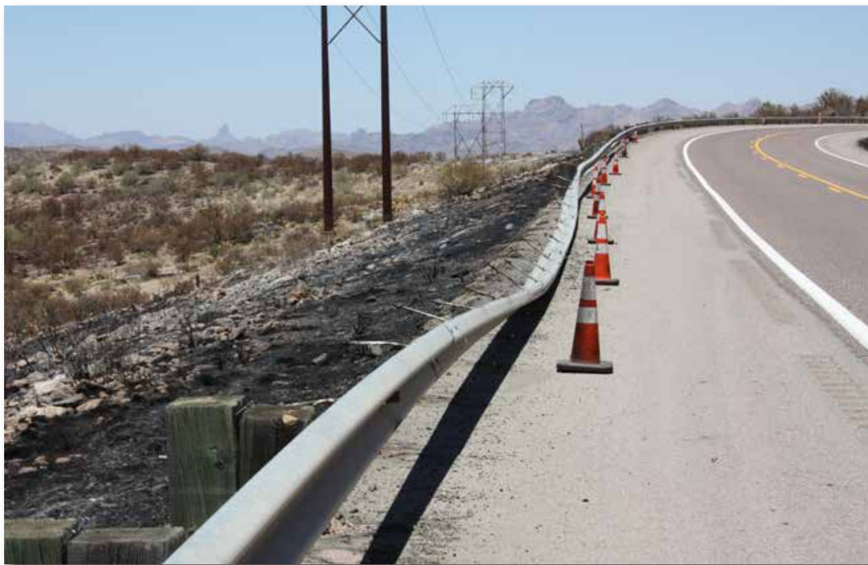
The guard rail posts were burned in several places on Hwy. 177 between Kearny and Superior due to the Telegraph Fire. James Carnes | Copper Area News
