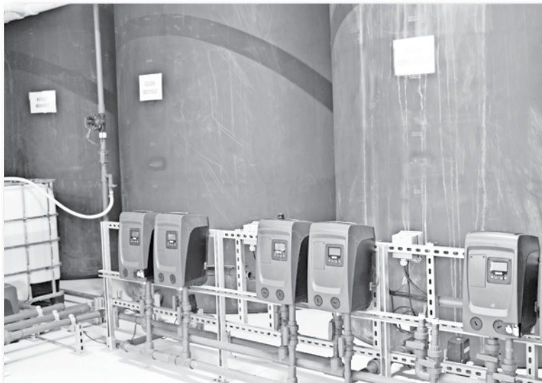
Part of the water recycling system at the Flower Mine in San Manuel.
