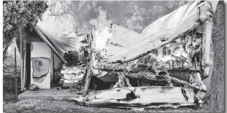
A fire destroyed two mobile homes at Top of the World at the end of April. Now volunteers are being sought to help clean up the mess.
