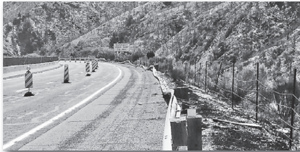
Guardrails on SR 87 south of Payson damaged by wildfire in 2020. Photo courtesy ADOT
