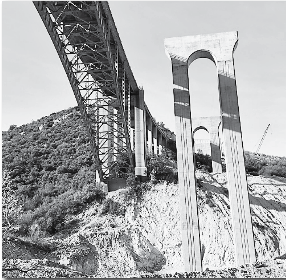
The new Pinto Creek Bridge is being constructed alongside the old bridge.
