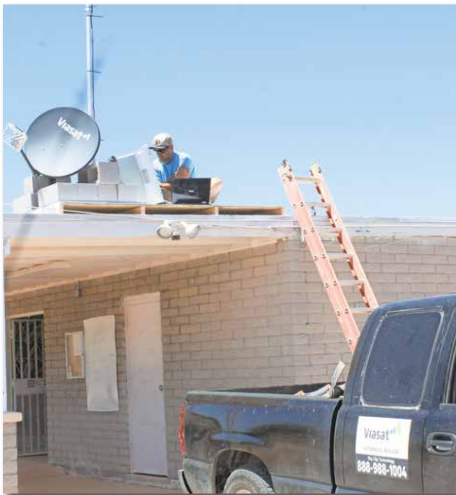
A technician with ViaSat installs a satellite WiFi receiver on the roof of the Mammoth Swimming Pool. The WiFi is for student use. John Hernandez | Miner
