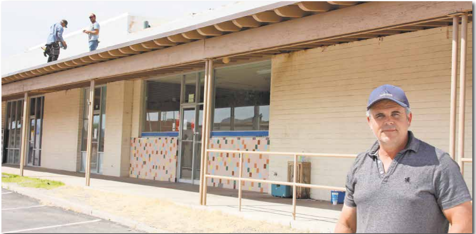
Workman just finished the front of the Kearny Retail Center from one end to the Cactus Mini Mart. The veterinarian’s office down the street also got nice coat of stucco. Workers are stuccoing the front of the Kearny Retail Center. James Austin with Sun State will be working on the roof soon. James Carnes | CBN
