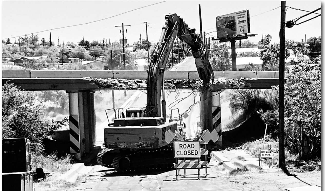
Stone Ave. is closed as the bridge is demolished to make way for a wider roadway. Drivers need to be aware of the detour.
