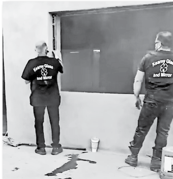
Kearny Glass & Mirror work to replace the windows in the front of Fly-N-Hi.
