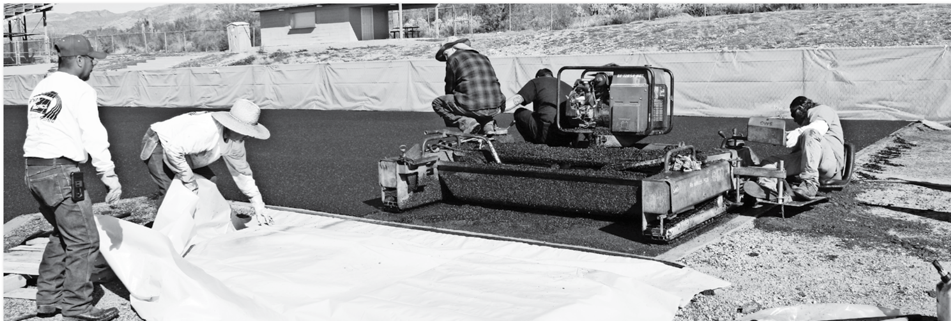
Construction is nearing completion on the Ray High School track. A crew from General Acrylics, Inc., puts the finishing touches on the track. The renovation is part of the bond election passed by voters.
