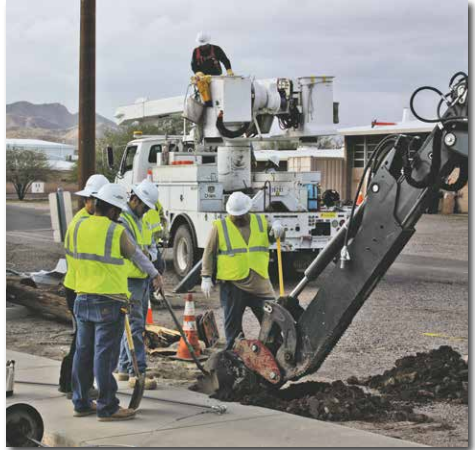
An APS crew replaces a damaged power pole at Ray Schools on Monday. James Carnes | CBN
