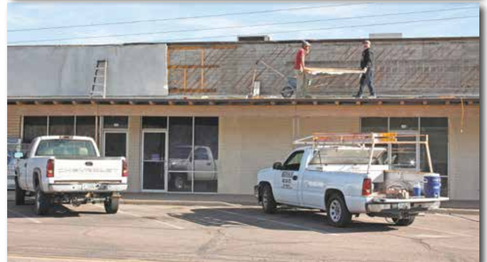
Old stucco from the front of the Kearny Innovation Retail Center is being removed this week. New stucco will be done soon. Doing the work are workmen from Construction Done Right, a local Kearny contractor.
