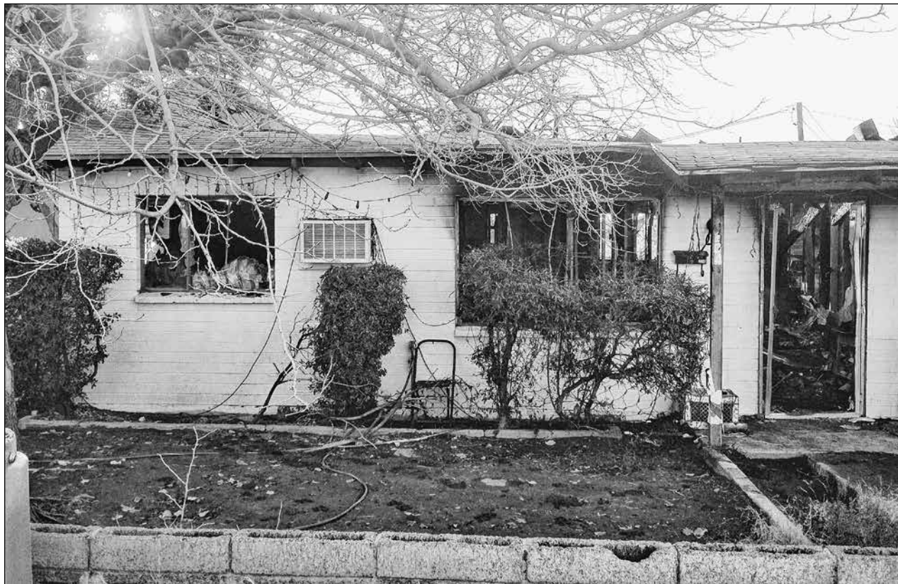
The home of Roy Chavez in the 100 block of W. Palo Verde, Superior, is a complete loss following a fire on Sunday, Jan. 5, 2014. (Mila Besich Lira photo)
