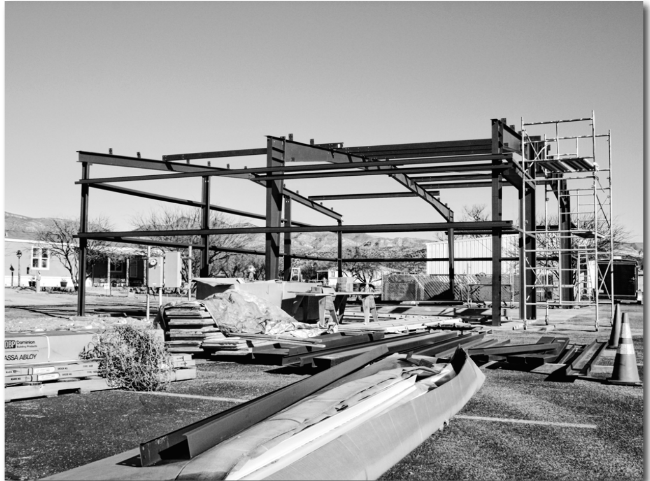
The new hangar is just bones now, but will soon be ready to house planes.
