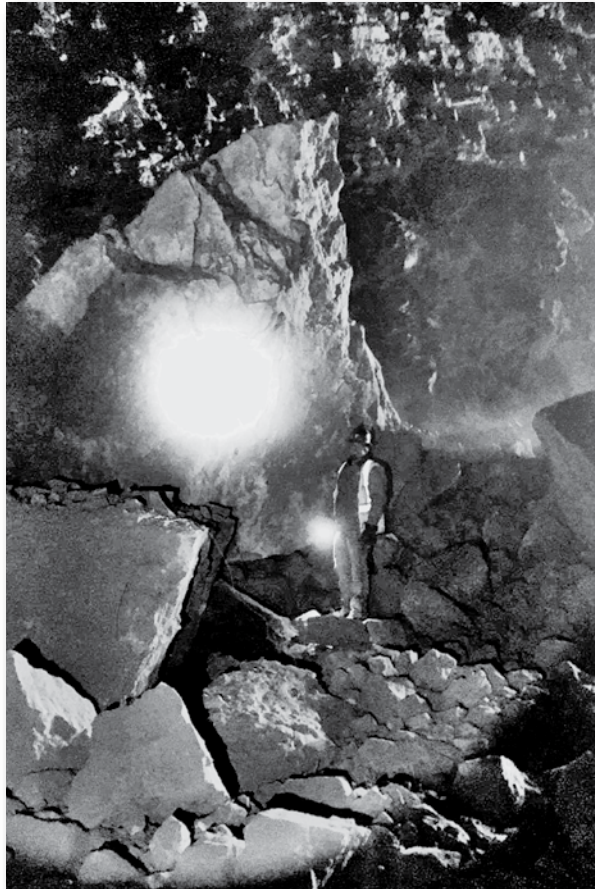
Blasting near Dripping Springs dislodged an 18-foot-tall monster boulder late last month prompting ADOT officials to move blasting to daylight hours.
