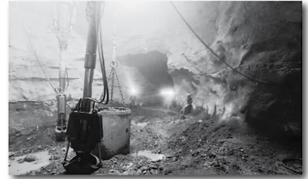
The last blast zone at the bottom of the shaft. Cementation | Submitted
