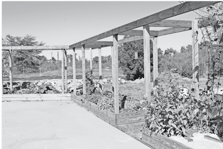
Volunteers built the raised planters, put in fencing and continue to give their time and labor to sustain the garden for the community to enjoy. John Hernandez | Miner
