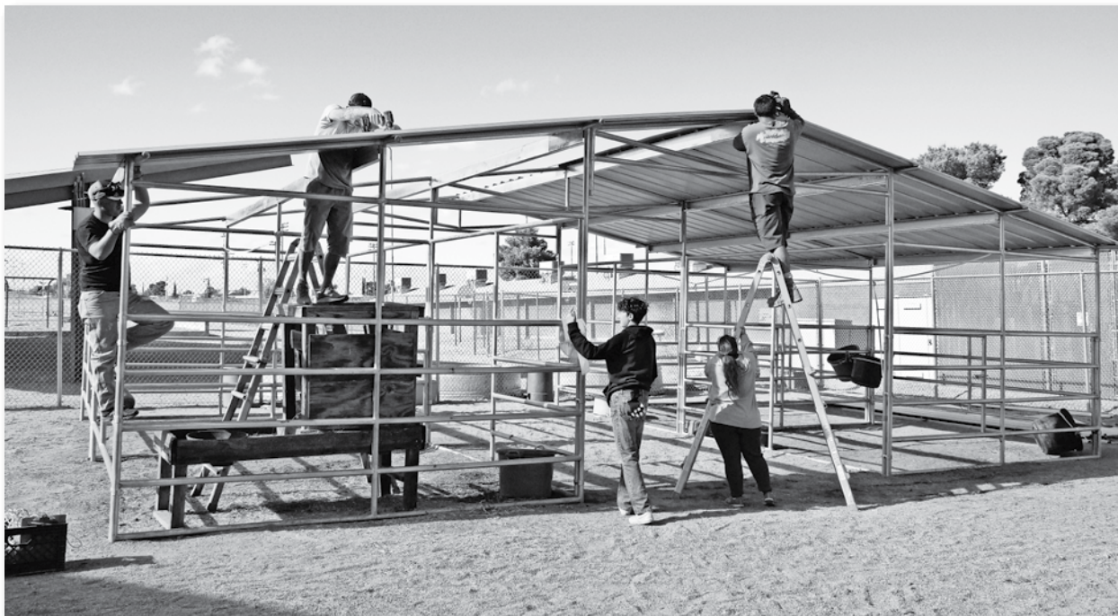
Volunteers work to place the roof over the mare motel at the Mammoth-San Manuel PreK-12 School. It will be used to house cows. Laurie Smalla | Submitted
