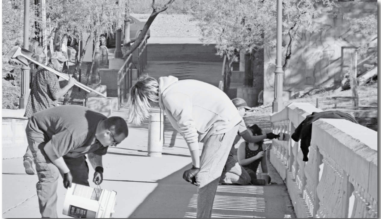
ASARCO employees paint the Historical Bridge in Winkelman. Vandals have painted graffiti on the bridge. Photo Courtesy Sylvia Kerlock, Town of Winkelman
