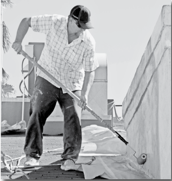
ASARCO's Paul Little paints the Kearny Police Department building. Sam Hosler | CBN
