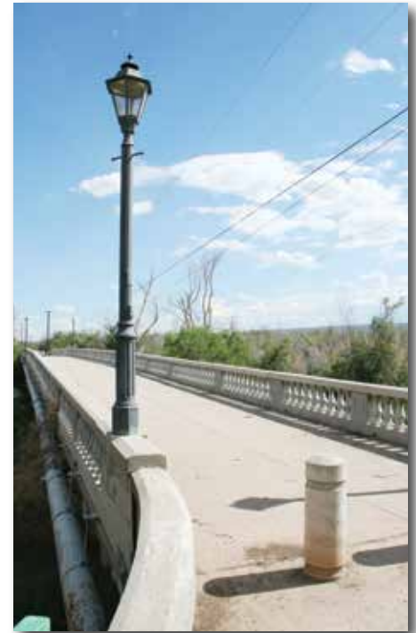
Historic Winkelman Bridge, designed by Daniel Luten and constructed in 1916, is owned by the Town of Winkelman. It was rehabilitated in 1999 by rehabilitation engineer Jerry A. Cannon and rededicated in 2016.
